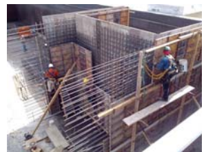
Baffle walls, City of Atlantic Beach Plant
